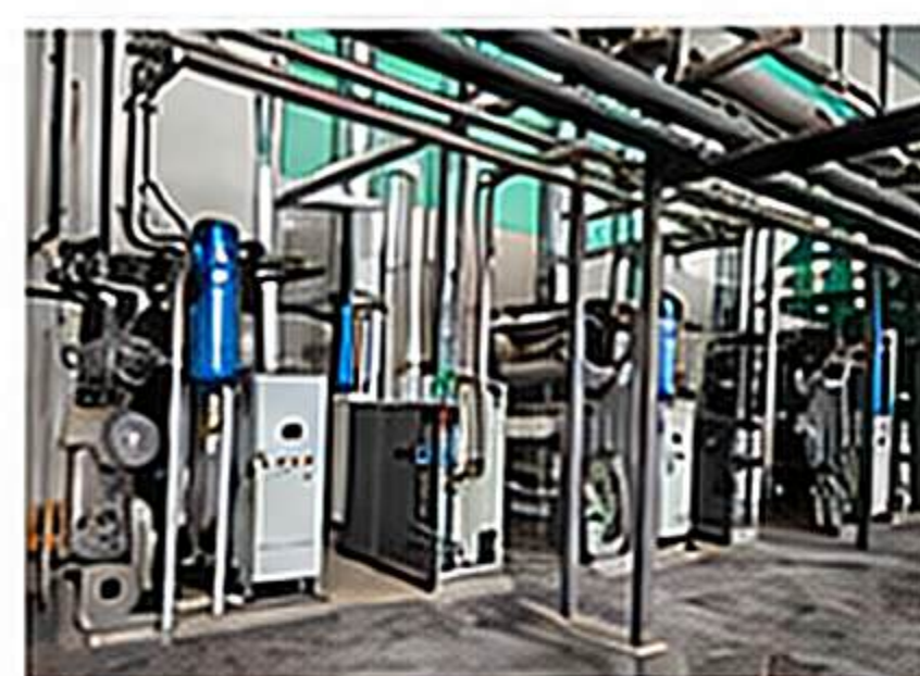
End User New Energy Materials Equipment Dual-tower heatless air dryer 2 sets (60 m³/min per set)
