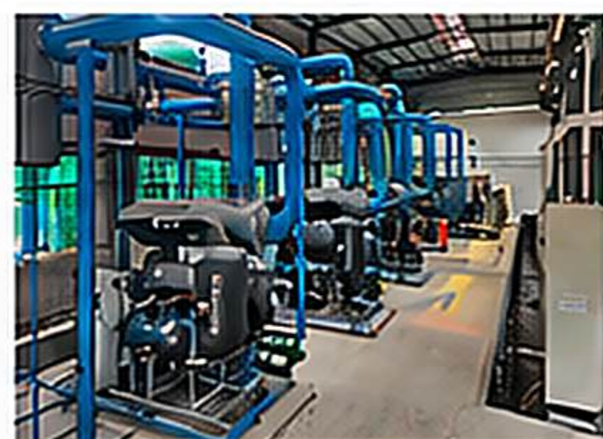
End User Chemical Plant Equipment Refrigerated dryer 8 sets (250 m³/min per set)
