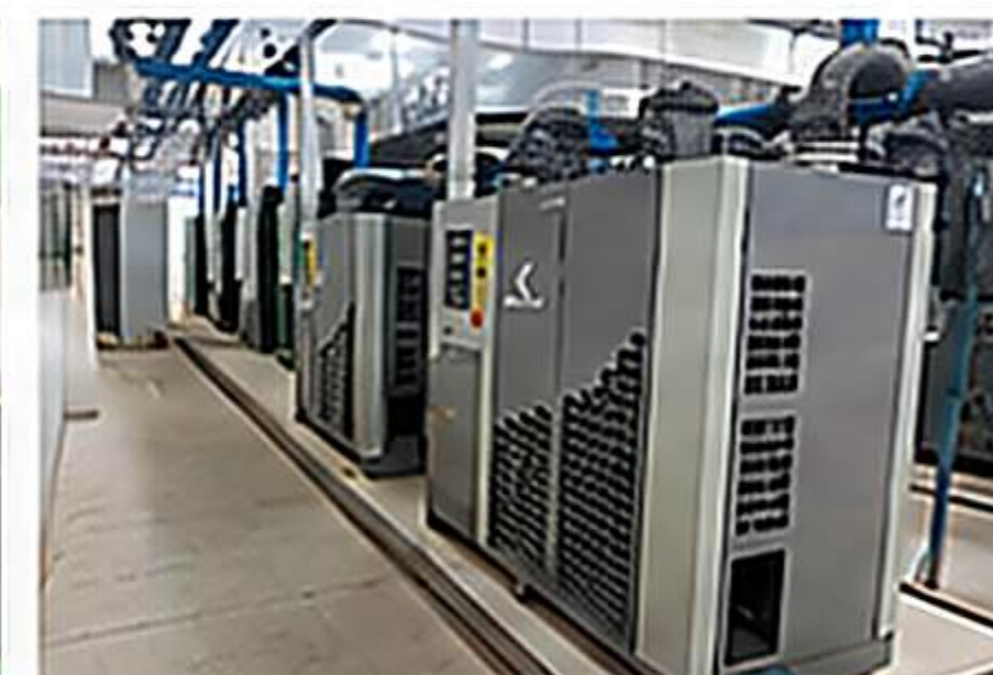
End User New Materials Equipment Refrigerated dryer 5 sets (55 m³/min per set)
