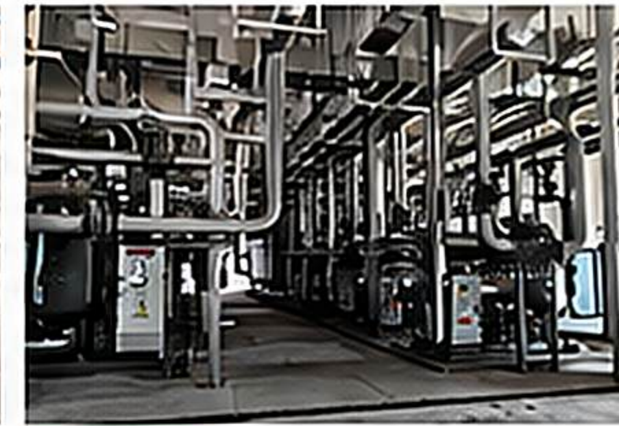
End User New Energy Industry Equipment Refrigerated dryer 5 sets (60 m³/min per set)
