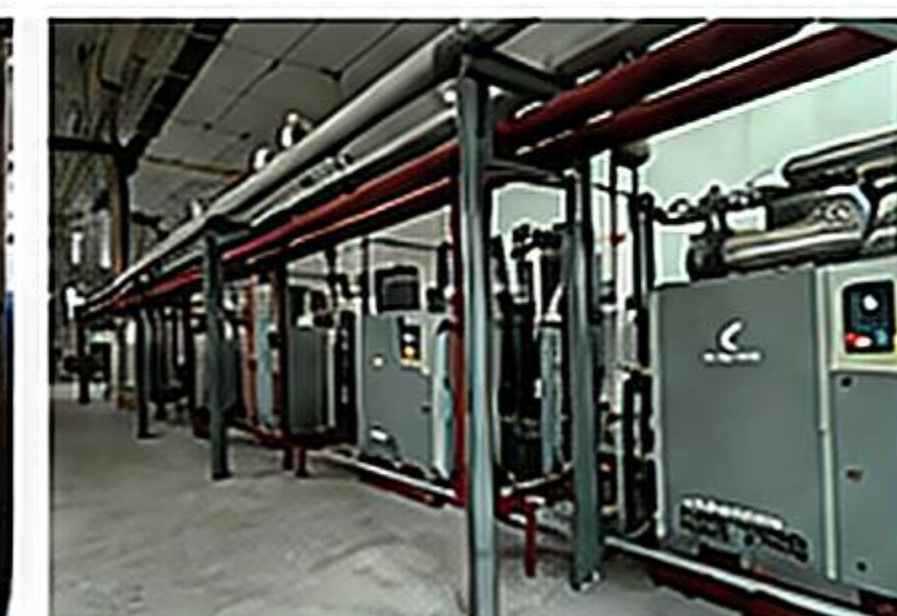
End User Pharmaceutical Industry Equipment Refrigerated dryer 10 sets (45 m³/min per set)
