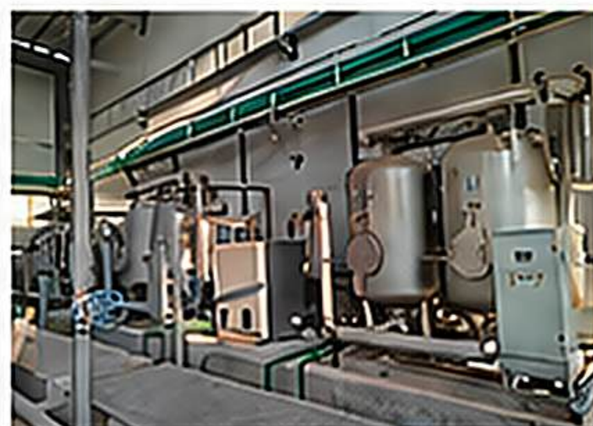
End User New Energy Materials Equipment Heatless dryer 9 sets (200 m³/min per set)
