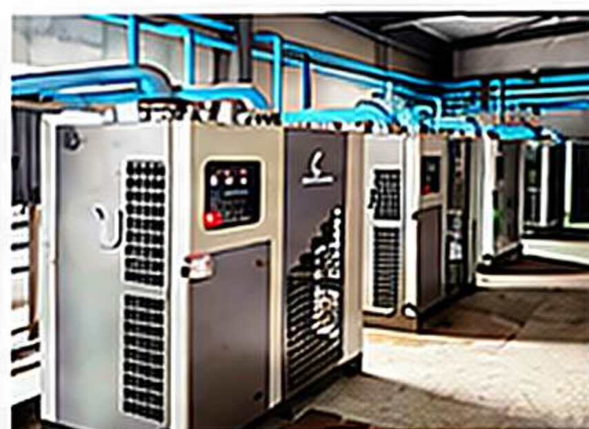
End User Water Treatment Industry Equipment Refrigerated dryer 5 sets (45 m³/min per set)
