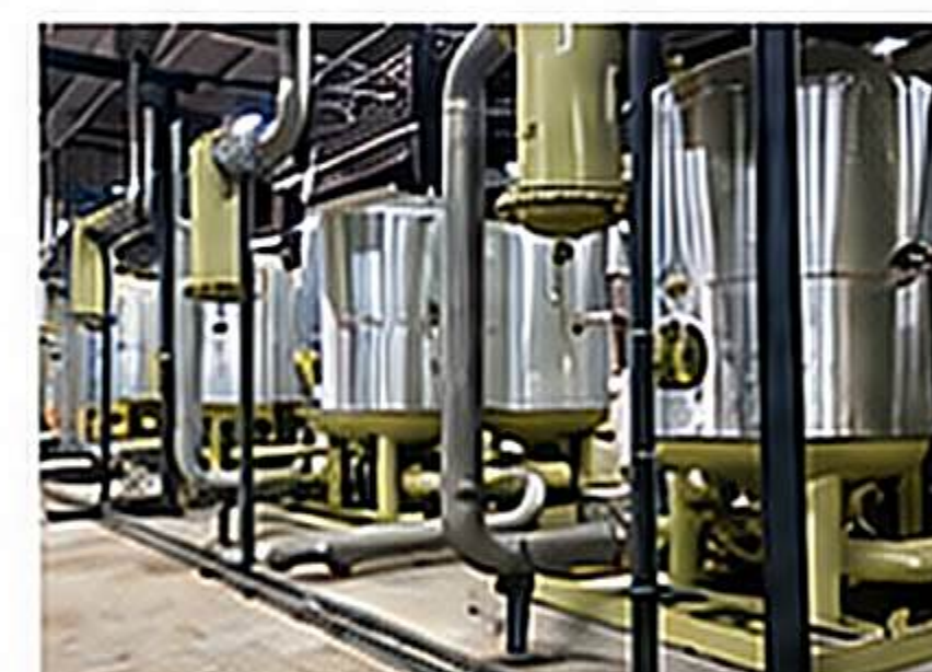
End User New Energy Industry Equipment Heatless dryer 12 sets (220 m³/min per set)
