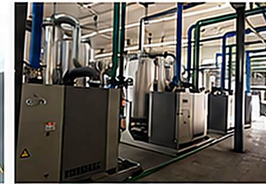
End User New Energy Industry Equipment Heatless dryer 3 sets (60 m³/min per set)
