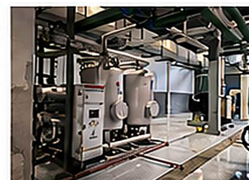
End User Battery Industry Equipment Heatless dryer 3 sets (85 m³/min per set)
