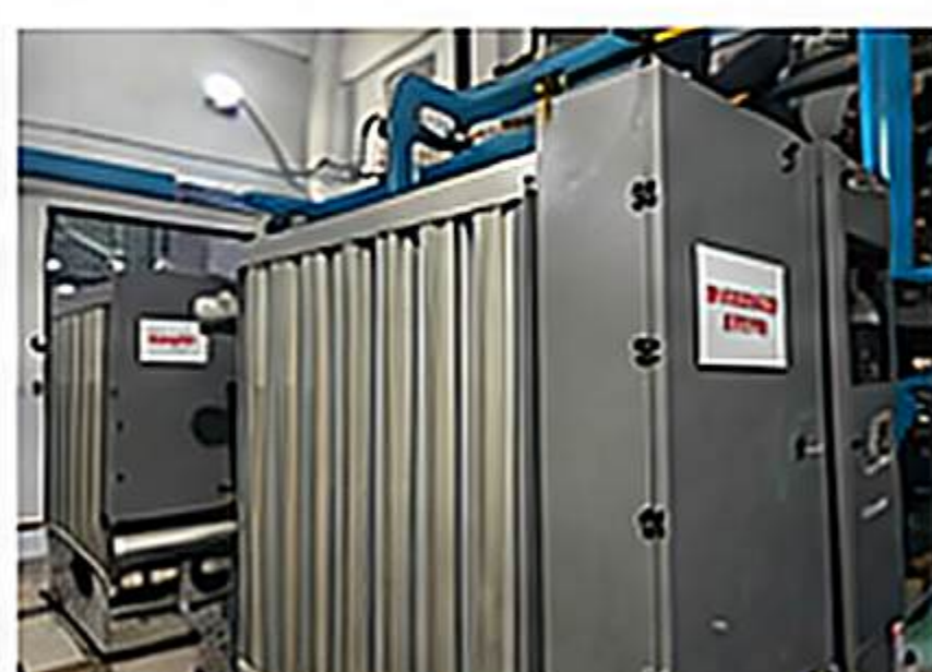
End User Power Plant Equipment Refrigerated dryer 2 sets (75 m³/min per set)
